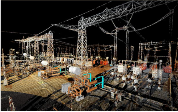
Figure 2: Hydropower substation 3D surveying and modeling of the Cahora Bassa dam in Mozambique. Point clouds have been coloured by projecting the photogrammetrically processed acquired images.
