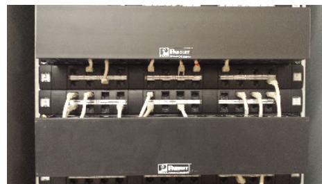
Figure 2: A section of the equipment in Figure 1.
