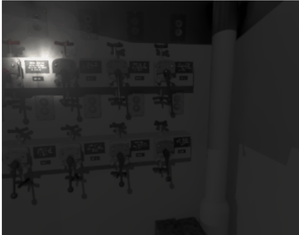
Figure 19. A simulation of a shipboard control panel under emergency lighting.
