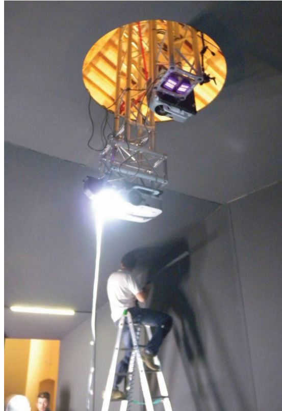
Figure 7a: Installation of infrared camera and videoprojectors for camera tracking on the ceiling
