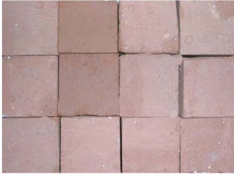
Figure 8: Wall consisting of small brick, two of the bricks are moist. The photo was taken with a digital camera
