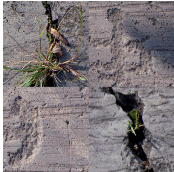
Figure 3: Exemplary problematic regions in the evaluation material. Grass (top left), shadow (top right), Horizontal scratches due to glacial polish (bottom left) and a deep crack (bottom right).
