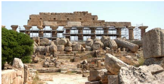
Figure 1: Temple C today. Fourteen columns on the North side, still in the position where they fell, were raised in 1925-1927 together with part of the trabeation.
