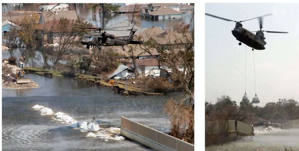
Figure 1.2 – Helicopters drop sandbags to seal the levee-breach in a trial-and-error approach. Initially, the sandbags are dumped too close to the breach and are washed away [132].
