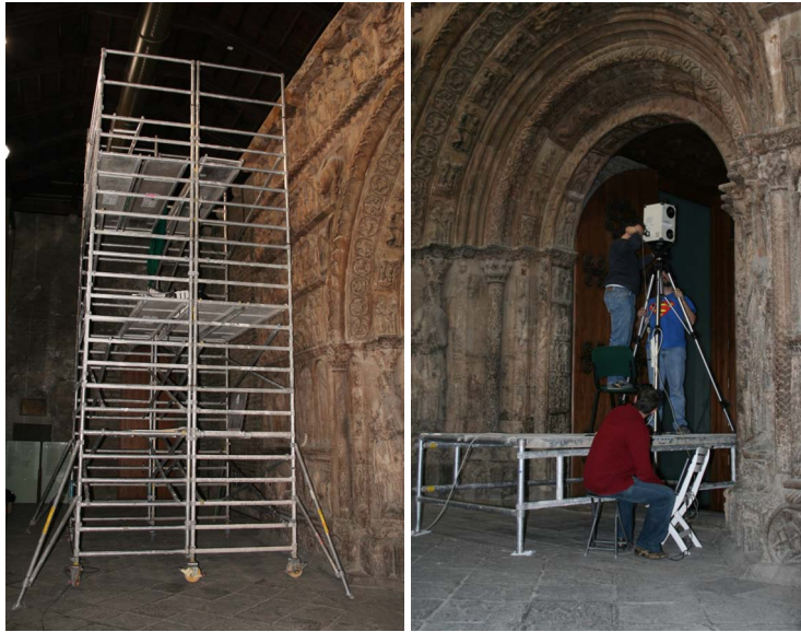
Figure 3.40: Left: the 7 meter high scaffolding used for acquisition. Right: a smaller scaffolding used for the acquisition of the internal part of the portal
