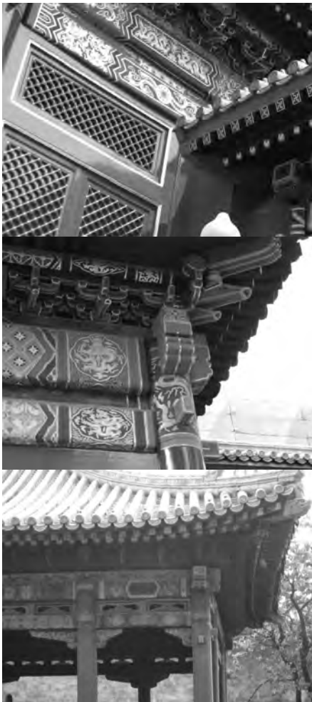
Figure 1. Three photos showing the colour decaying on historical buildings in the Forbidden City, Beijing, China. Top: a recent repainting (presumably with the original colours); middle: colours started to decay; and bottom: significant colour fading.
